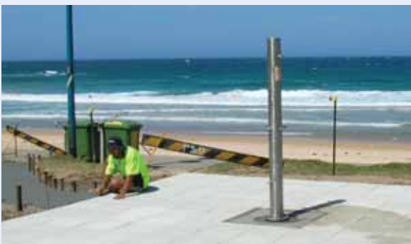
Low flow shower with water permeable pavers located at Queenscliff. Source: Manly Council
